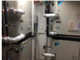
Water Cooled condensing units located in a mechanical room.
